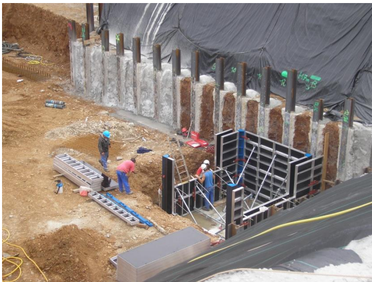
CAZES parking souterrain CAHORS
